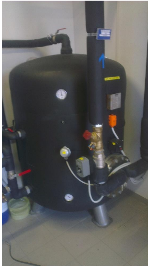
1000 L hot water tank.
